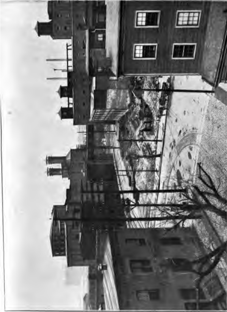
Photograph kindly furnished by Newark City Plan Commission Illustration No. 7. —The widening of Front street, Newark, N. J., shown herewith under construction, is characteristic of several street openings now necessary in St. Louis.
